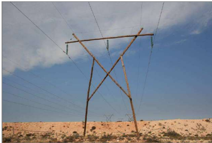
Figure 2.2 Example of an existing 132 kV transmission line (taken 29/09/2011)
