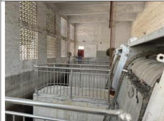
Xiangyang storm water pump station
