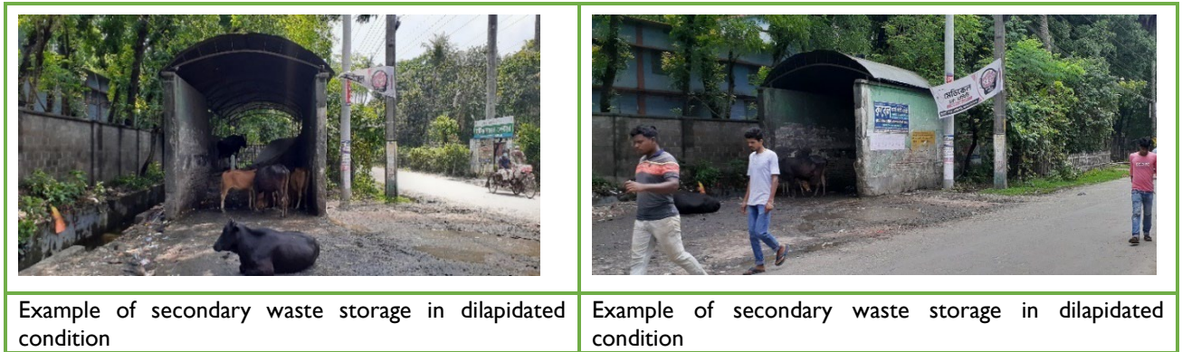
Example of secondary waste storage in dilapidated condition
