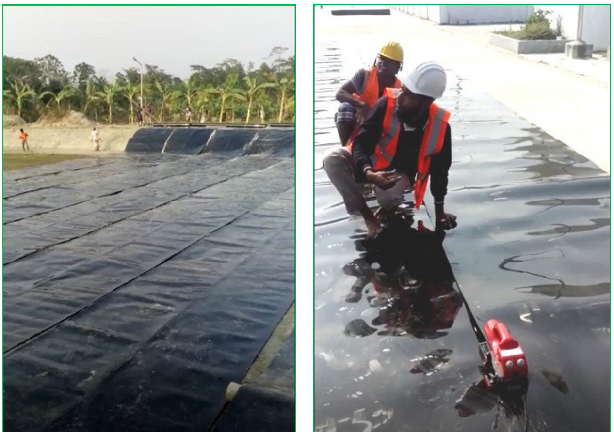
Figure 3-36: 1.5 mm thick HDPE Liner on top of the Clay Layer shall be used to manage leachate
