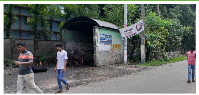
Secondary Waste Storage in Dilapidated Condition
