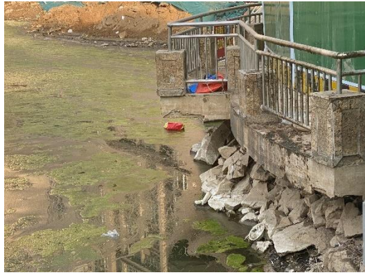
Damaged Dihu Bridge
