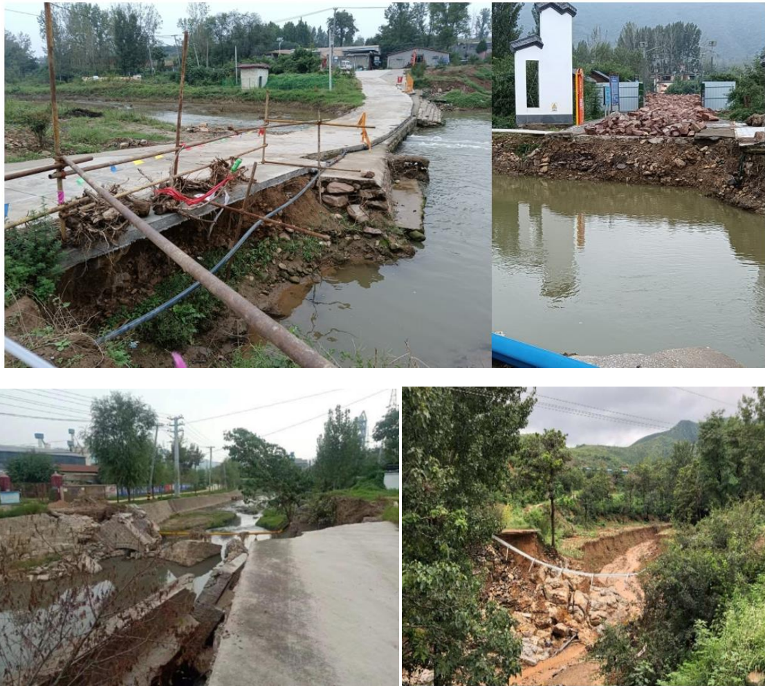
Rural roads destroyed by the flood
