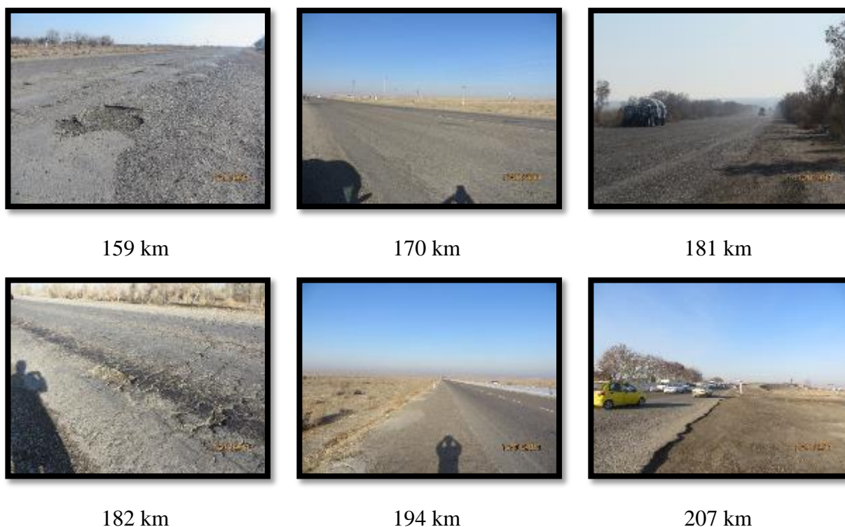
Figure 4.1: Current condition on different sections of the A380 road
