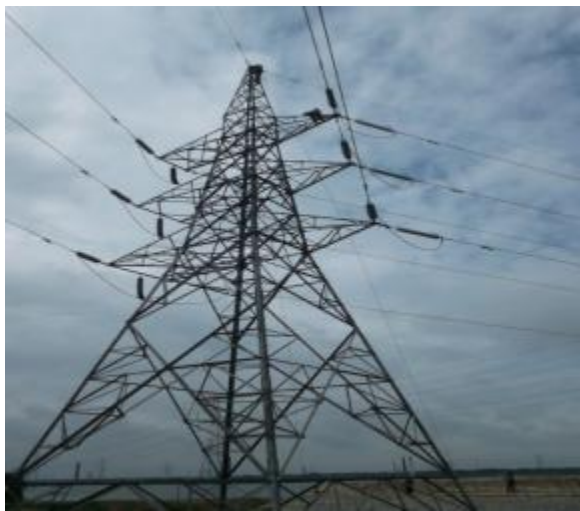
Figure 3.5: Angle Tower (Tension Tower)
