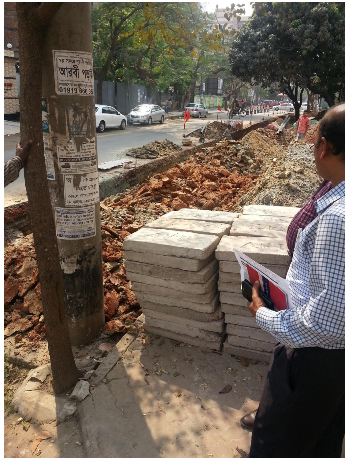
Figure 5.2: Underground construction of 33 kV lines showing temporary material stockpiles and safety markers. Stockpiled RCC slabs, which are placed on back-filled trenches, are visible in the foreground.
